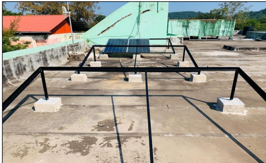
Stands used for supporting the solar panels
