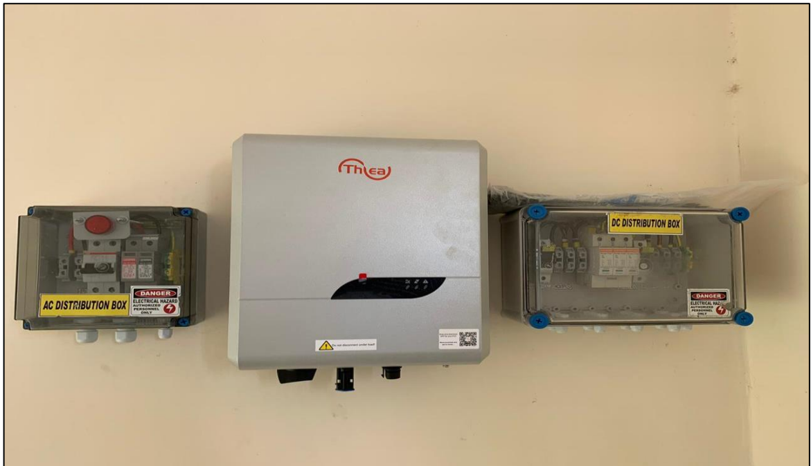
(L to R) AC Distribution box, solar inverter, DC distribution
