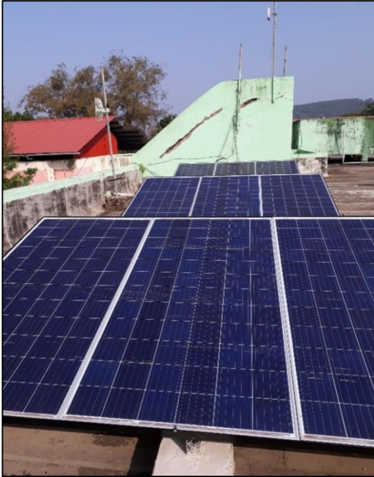
Mounted solar panels
