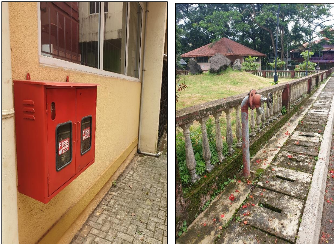
Fire hose box placed outside the Quad area in A-block and water facility
