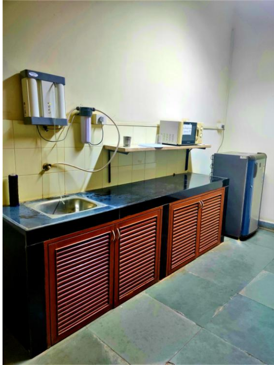
Drinking Water and Filter
