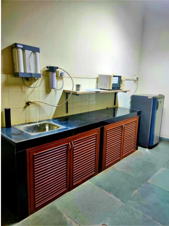
Drinking Water and Filter
